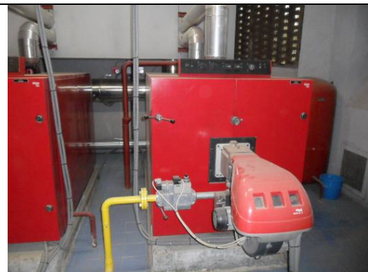
Calderas Gas natural
