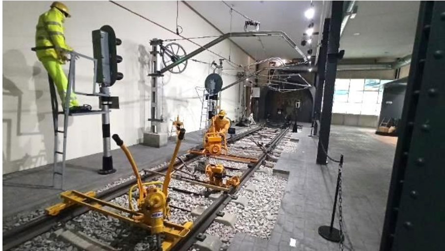
Image 27: Interior of the infrastructure room
